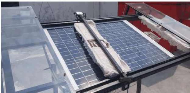
Figure 15. Solar Panel Surface Drying Process
