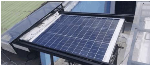
Figure 14. Wet Solar Panels
